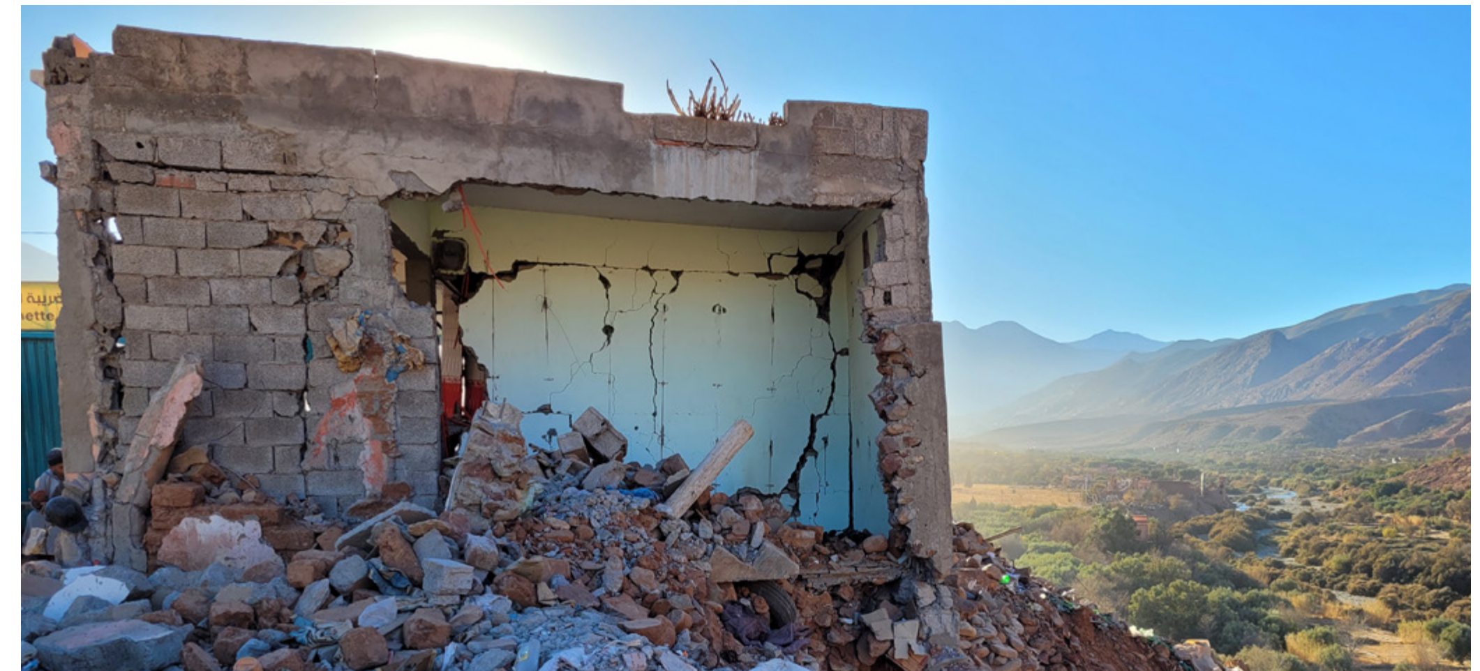
Exhibit 28: Examining the Earthquake Damage in Talat N'Yaaqoub
